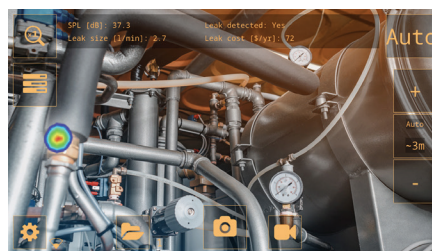
Compressed Air Leak
